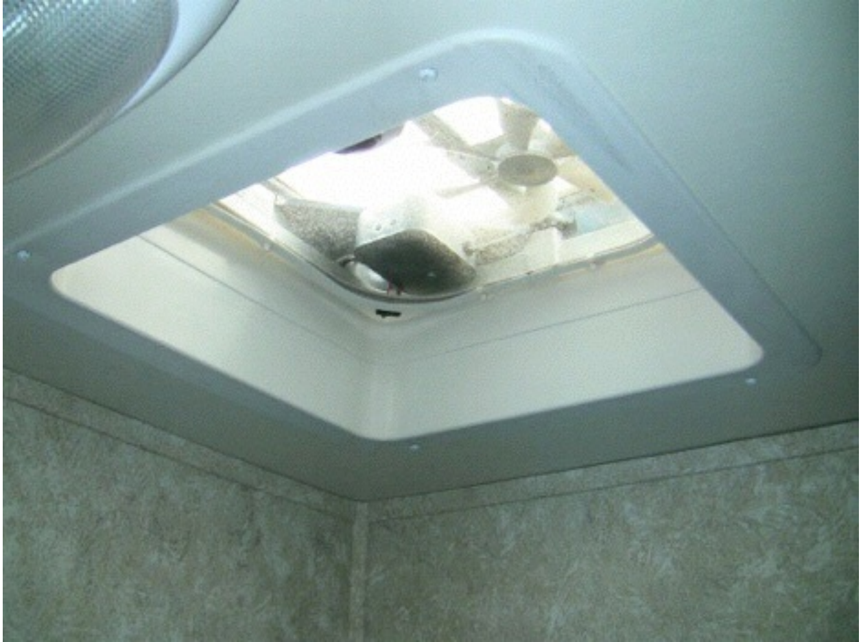
RV Bathroom Vent Fan and Switch
