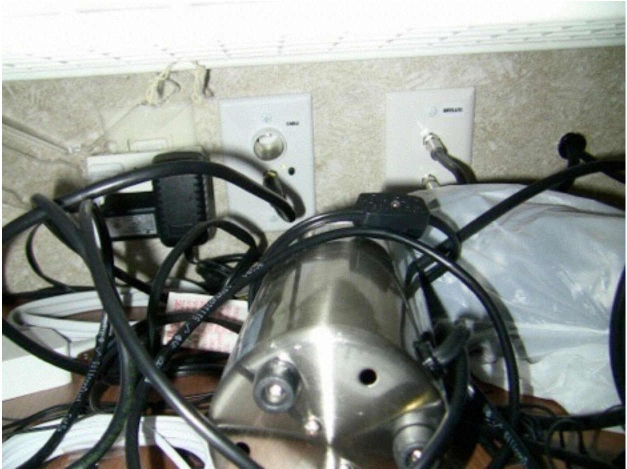
RV Antenna Cable Switch and RV Antenna amplifier
