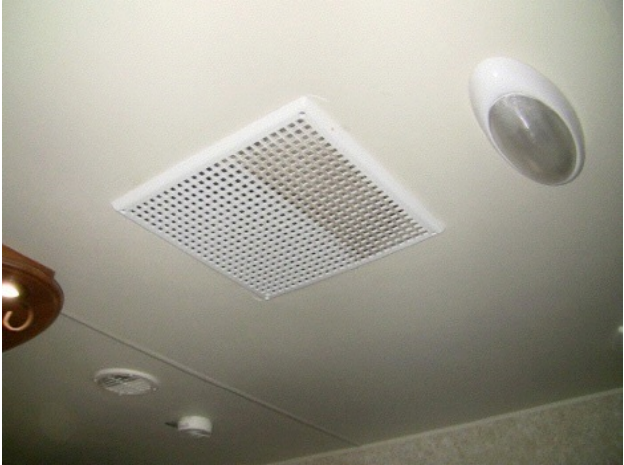
RV Air Conditioner and Return Vent
