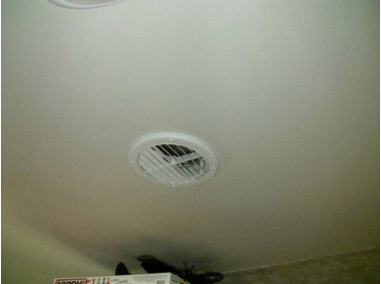
RV Air Conditioning Outlet Vent
